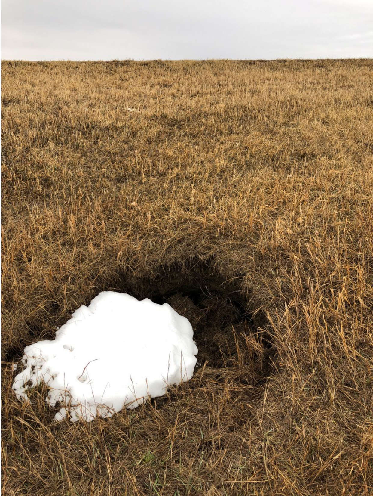
Figure 1: A sinkhole in the ditch of Lehigh Road that formed in the spring of 2022. Drilling near this sinkhole located additional underground mine voids.
