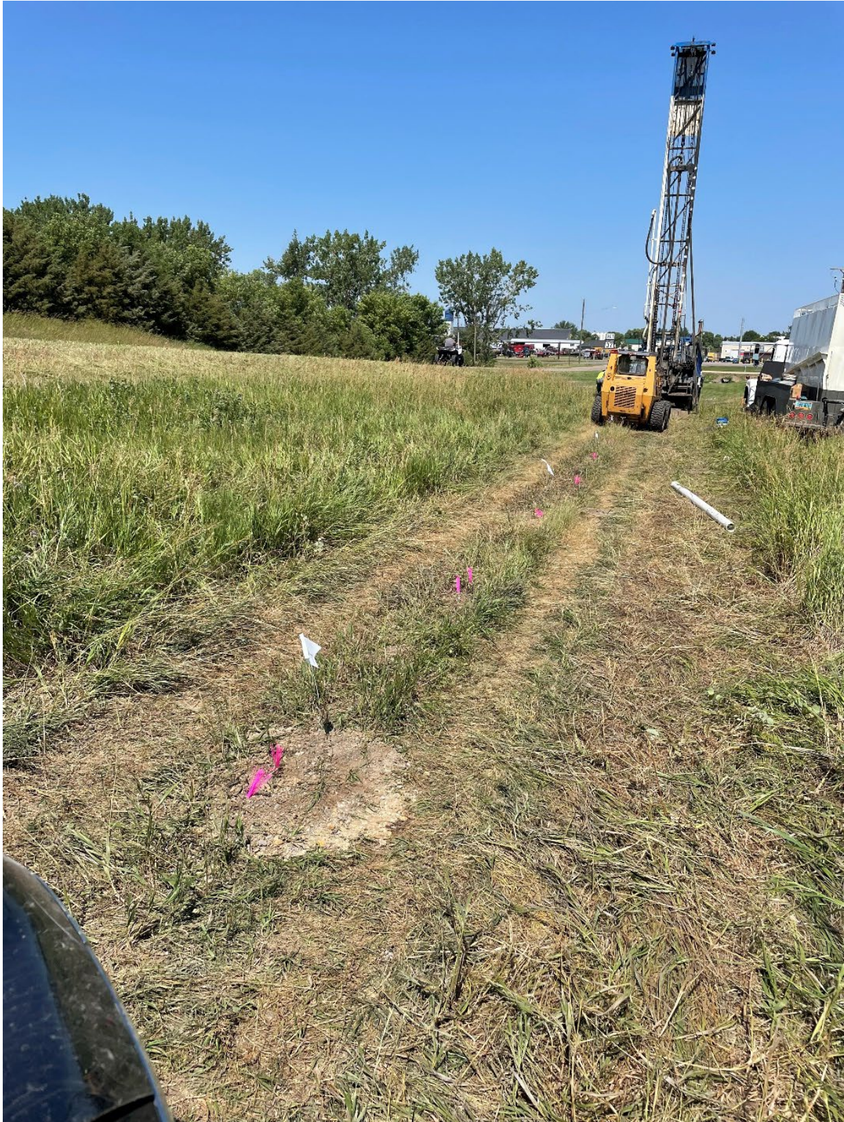
Figure 4: The drill rig is facing north in the east ditch of McLean County Highway 15. Buildings in Garrison can be seen in the background.
