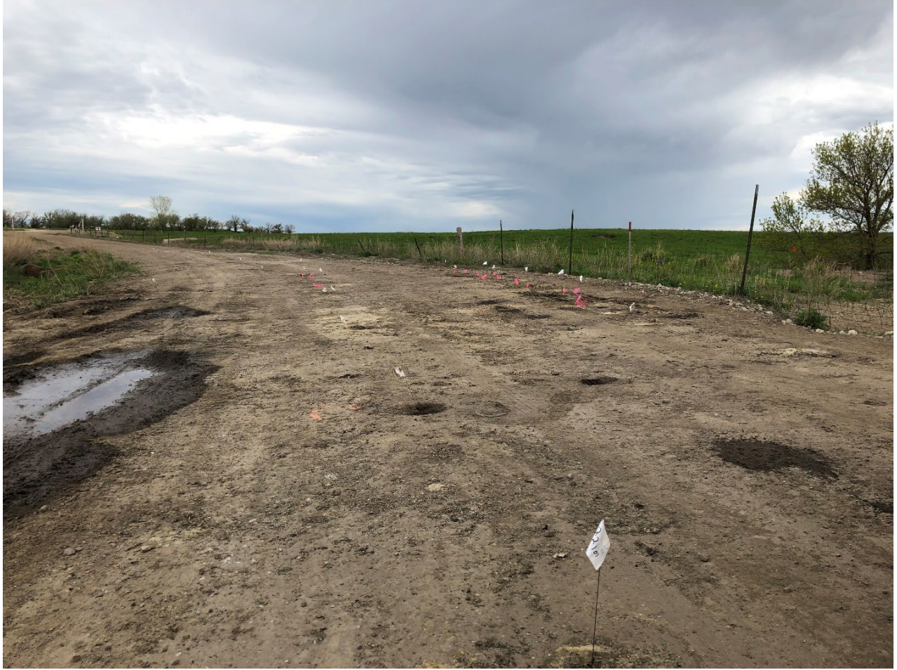
Figure 2: The white pin flags indicate drillhole locations. The pink whiskers indicate a drillhole encountered a mine void. Voids are cased with schedule 40 PVC pipe. This area is a driveway to an industrial business off Lehigh Road.
